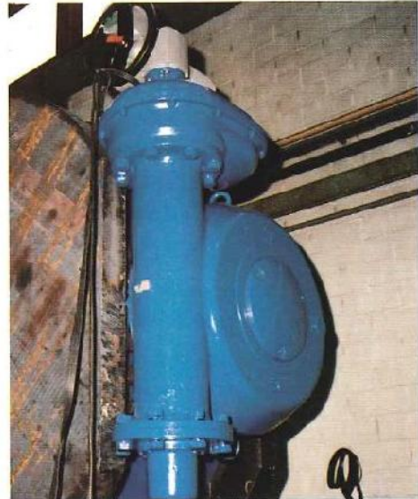
Worm gear reducer with electric actuator under testing
